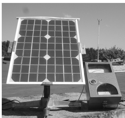
Fig. 1. Photovoltaic panel PVM10/12PF in fixed position with power measuring device
